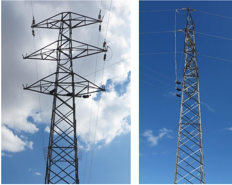
Figure B.5. No.127 tower (Deformation of the tower cage)
